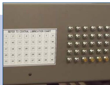
Central Point Lubrication
